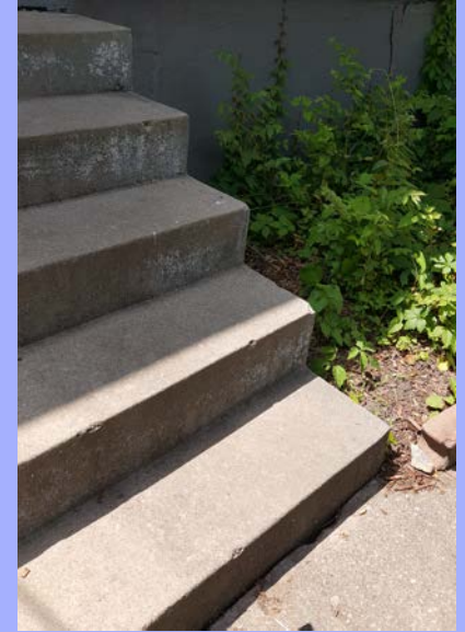
Loose or lack of railings
