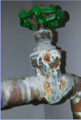
Corrosion on pipes
