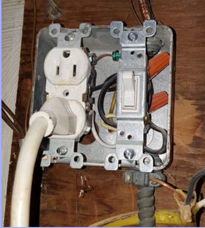
Uncovered Junction Boxes
