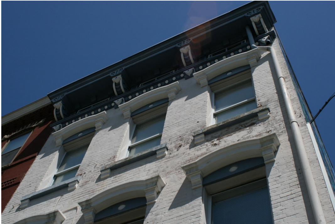
West Façade – Peeling Paint
