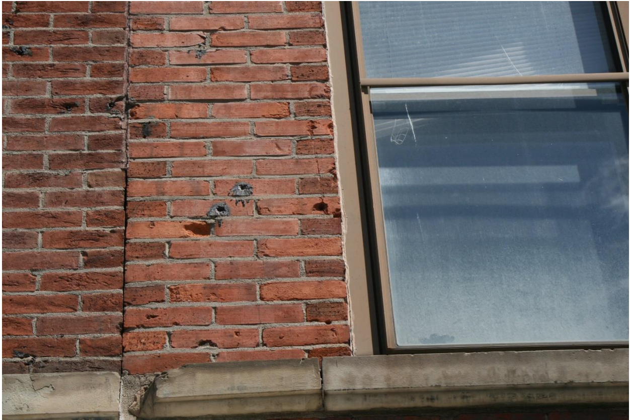
West Façade – Spalled Brick
