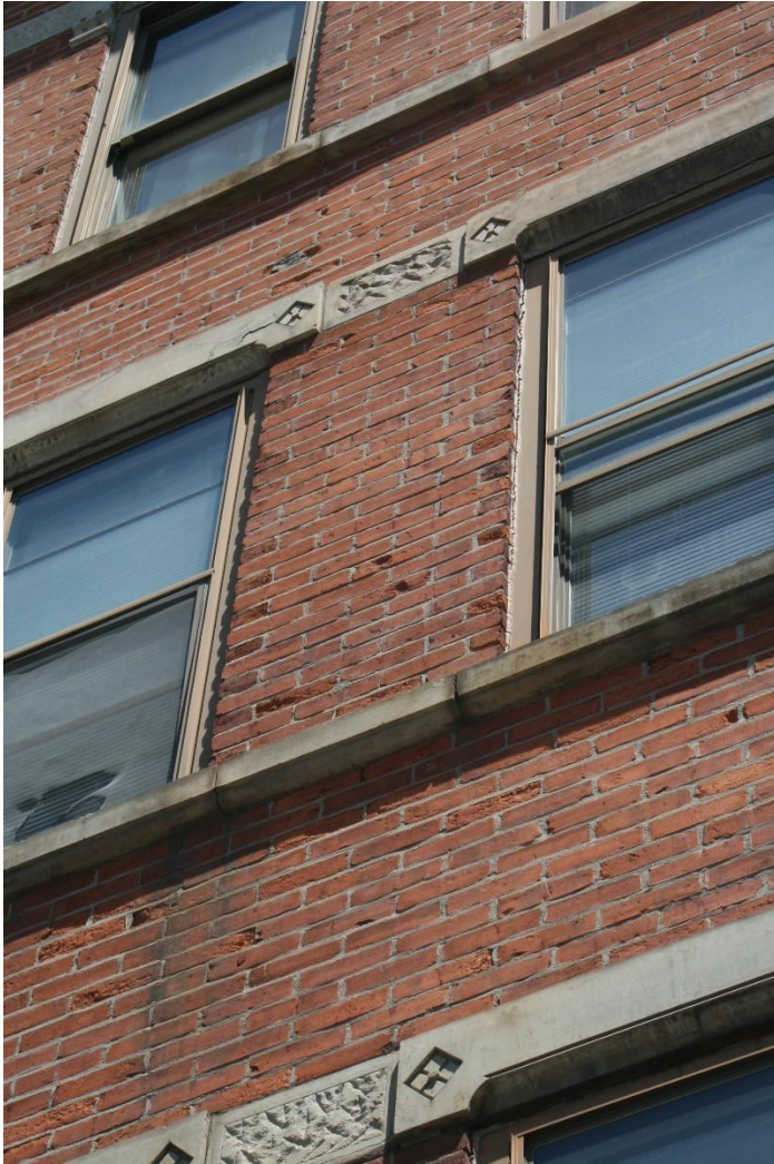
West Façade – Cracked Stone Header / Spalled Brick
